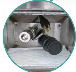
Exterior fill box for deliveries and pickups
