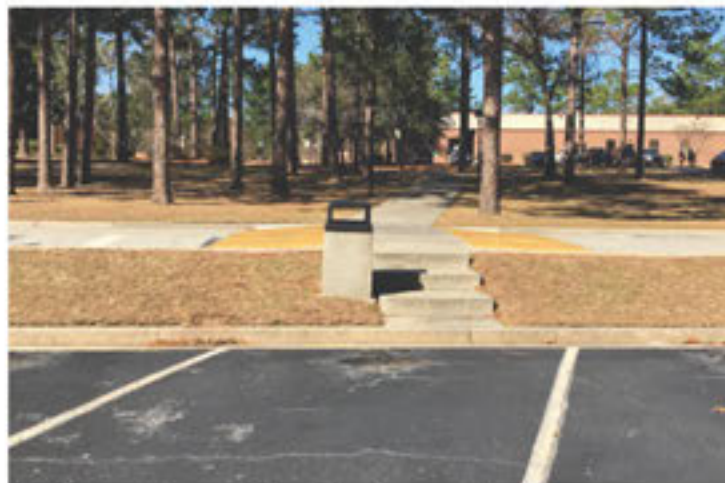
No clear path to stairs leading from parking lot.
